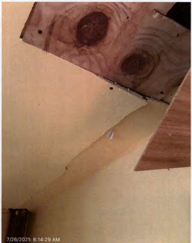
Collapsing ceiling in front entryway
