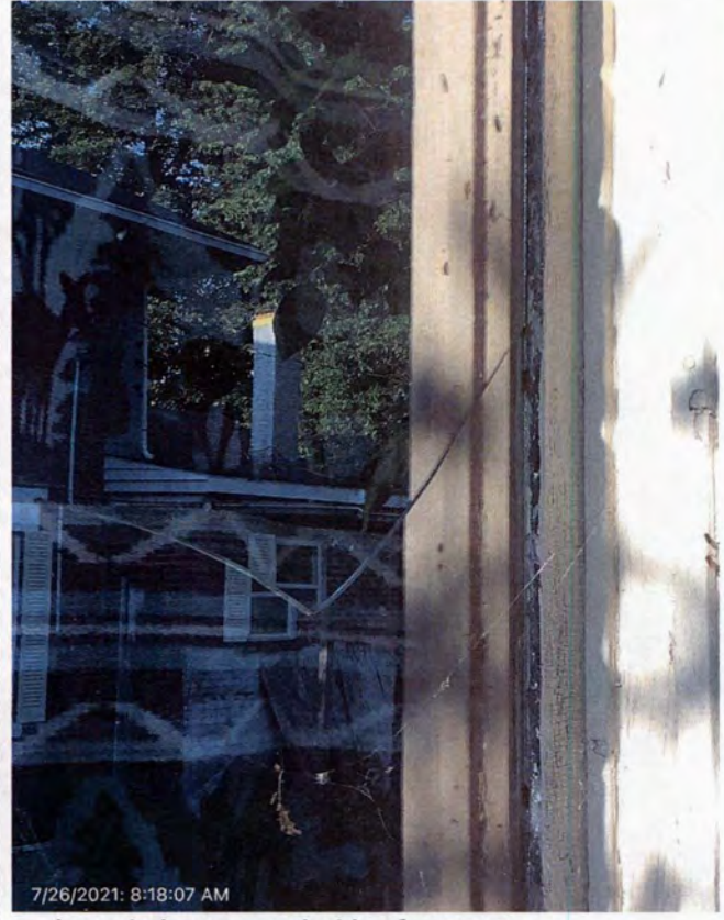
Broken window on north side of property
