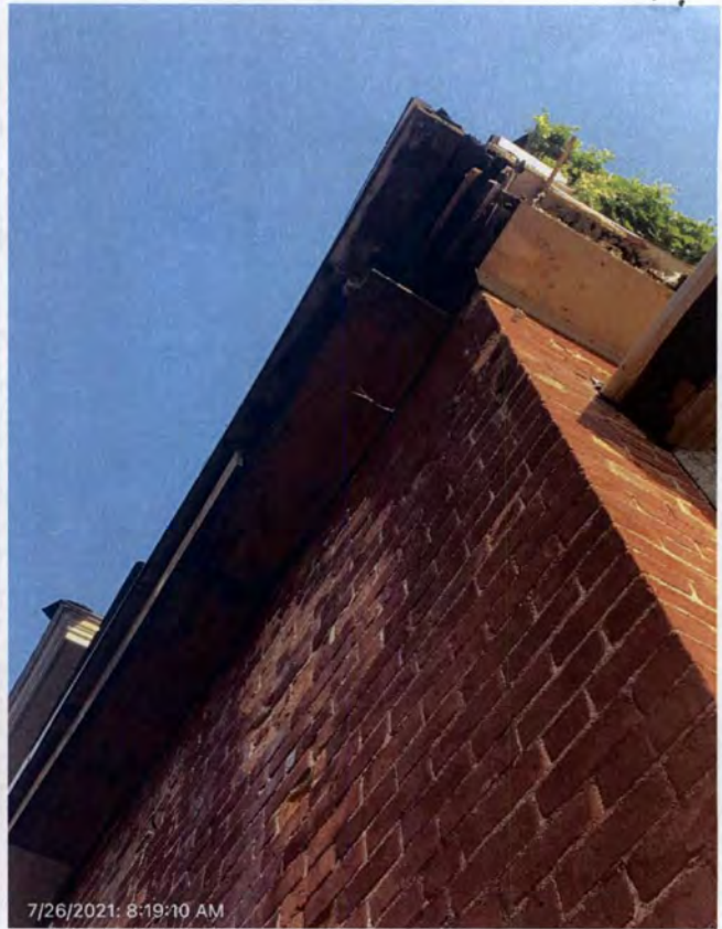
Attempted repairs to fascia board at front of property
