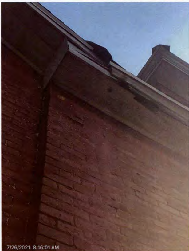
7/26/2021 8:16:01 AM Deteriorating fascia board at rear of property
