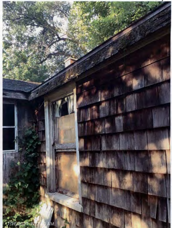
Deteriorating fascia board at rear of property
