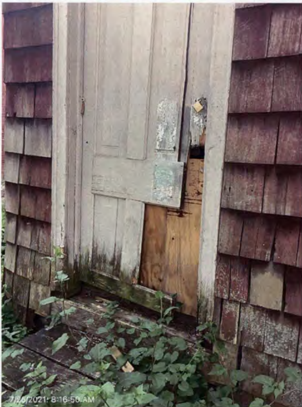
Door in disrepair at rear of property
