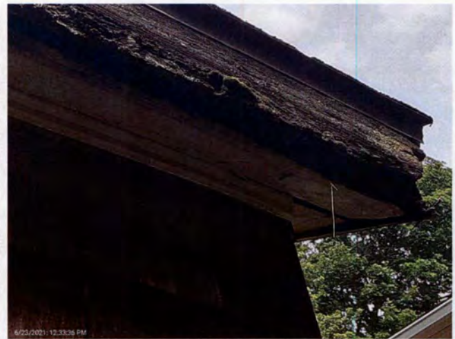
Deteriorating fascia board at rear of property
