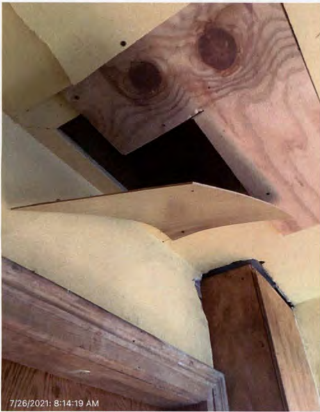
Collapsing ceiling in front entryway
