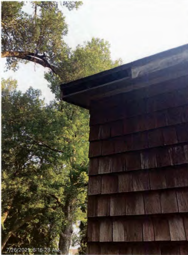
Missing fascia board at rear of property
