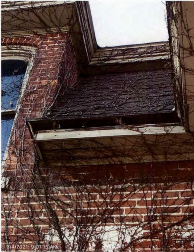
Missing wood trim at rear of property
