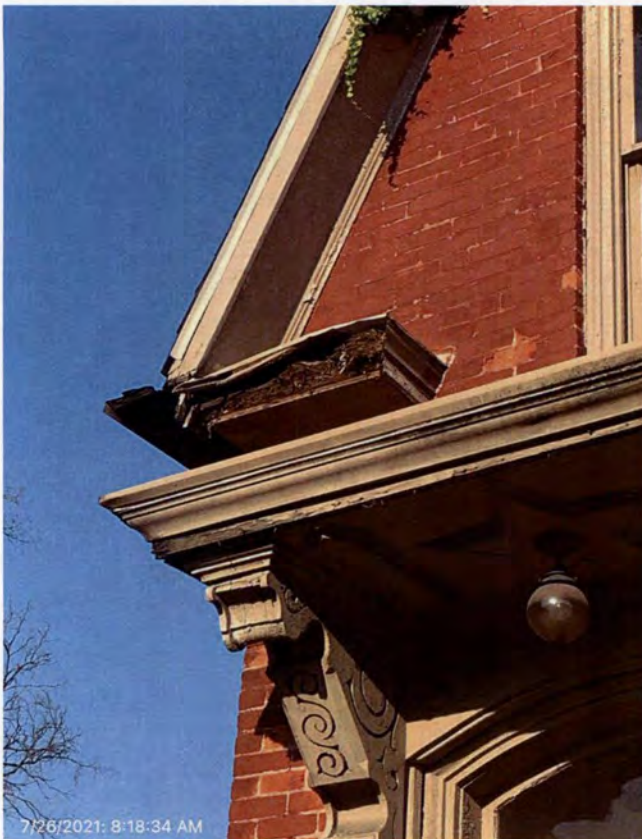
Deteriorating trim at front of property
