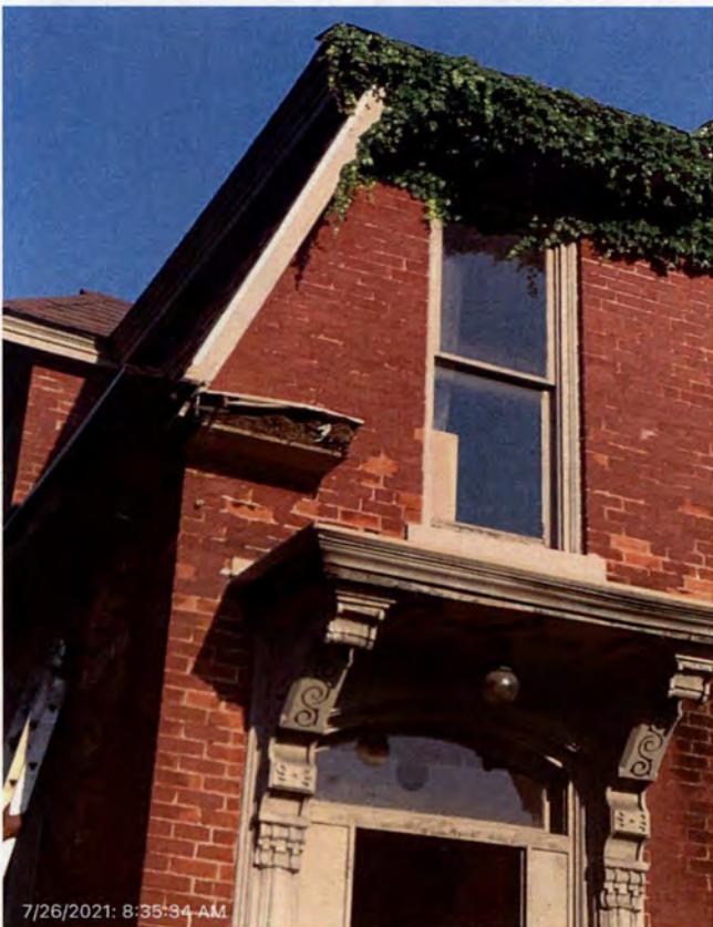
Deteriorating wood trim at front of property
