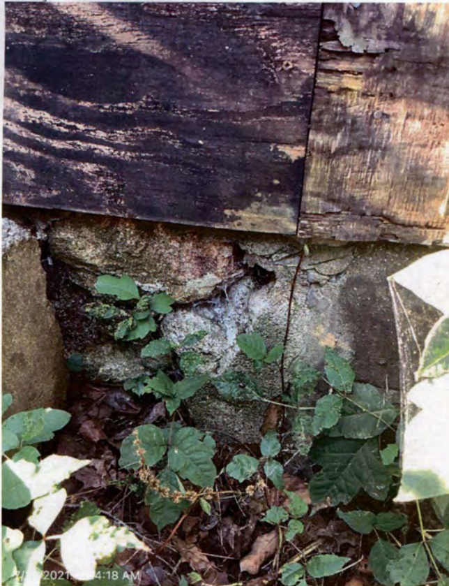
Gaps in foundation on south side of property
