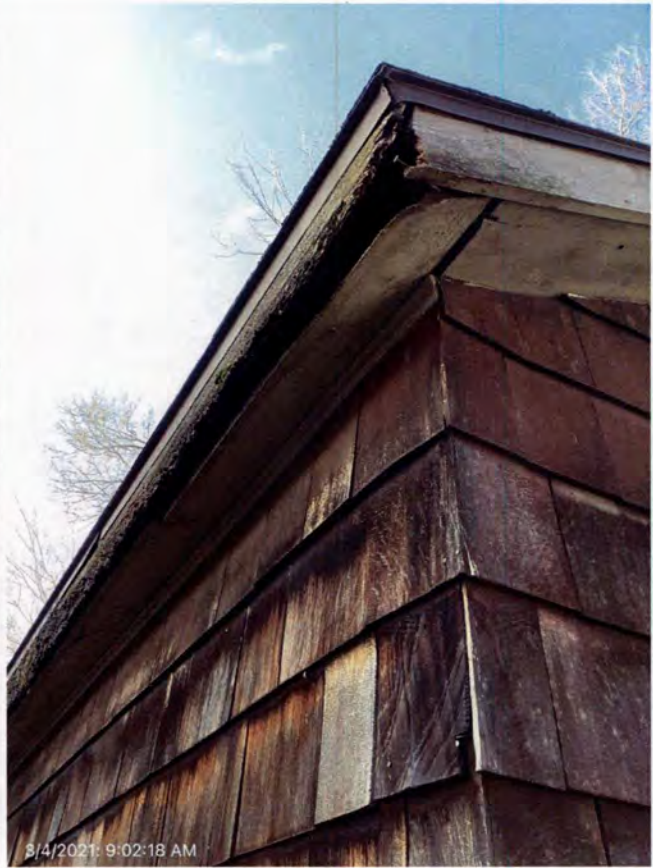
8/4/2021 9:02:18 AM Deteriorating fascia board at rear of property
