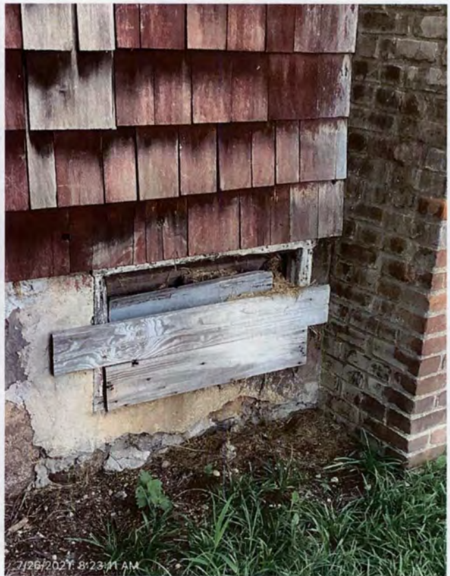
Improperly covered basement hatchway/ window
