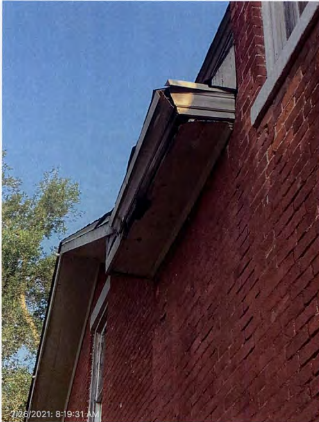
Loose fascia at side of property
