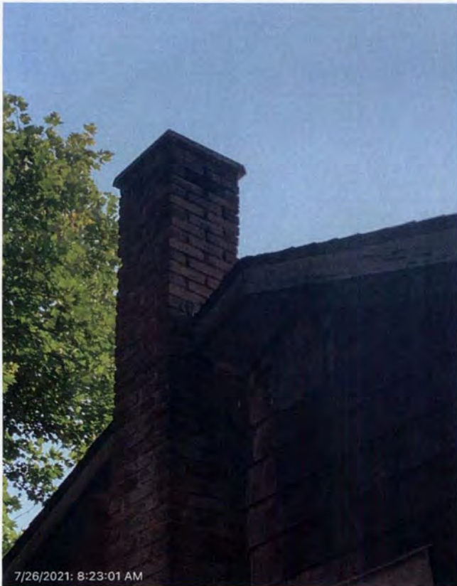
Damaged chimney at rear of property
