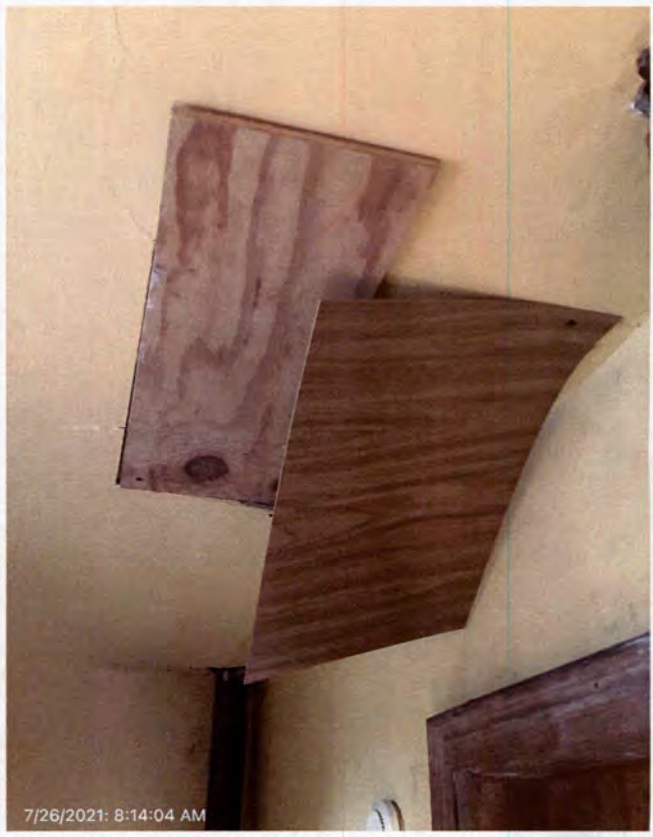
Collapsing ceiling in front entryway
