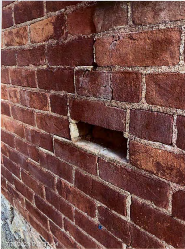
7/26/2021 8:15:37 AM Deteriorating exterior wall on south side of property
