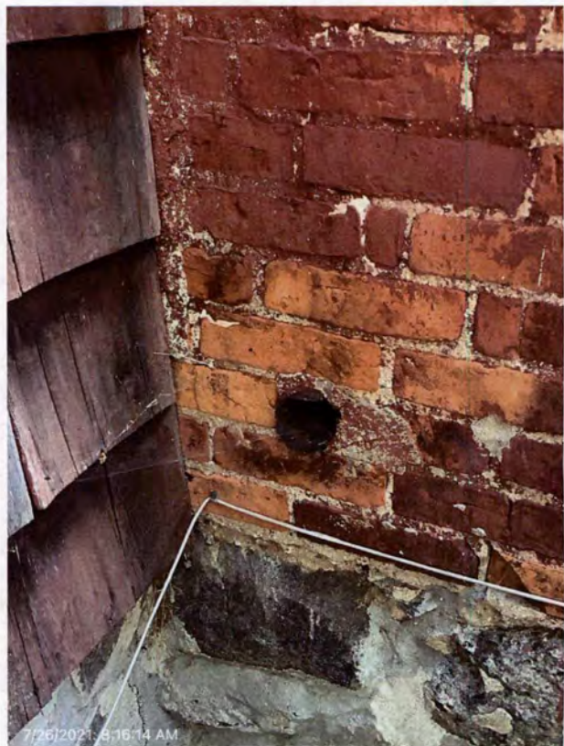
7/26/2021 8:16:14 AM Hole in exterior wall
