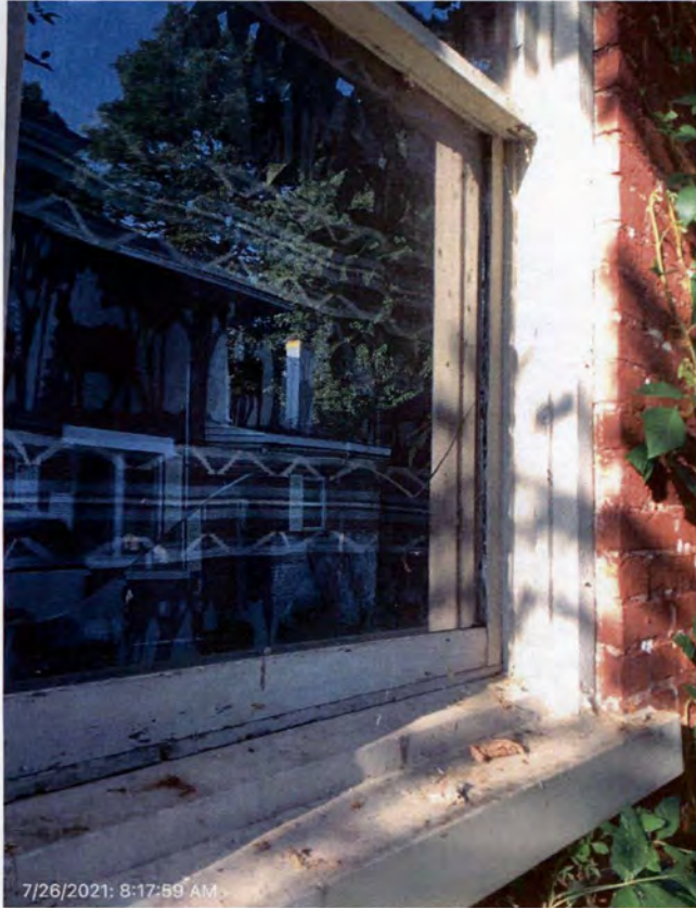
Broken window on north side of property
